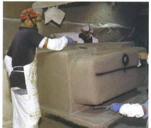
Bubbles or voids in the fiberglass layer will weaken tub-shower walls, so fixtures are thoroughly rolled out by hand after they are sprayed.
